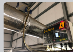
Gas Flow Monitoring
